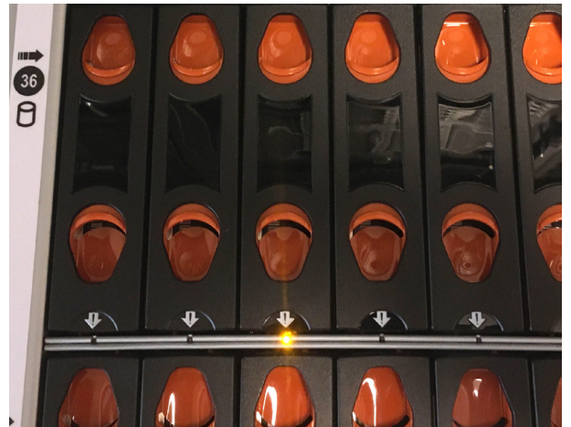
Indication of faulty drive in extension chassis
